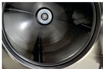
Gambar 5.13. Bagian tabung washing machine Sumber: Hotel Eastparc Yogyakarta, 2018
