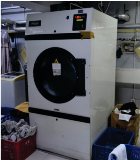
Gambar 3.14. Drying Tumbler Sumber : Hotel Eastparc Yogyakarta, 2018
